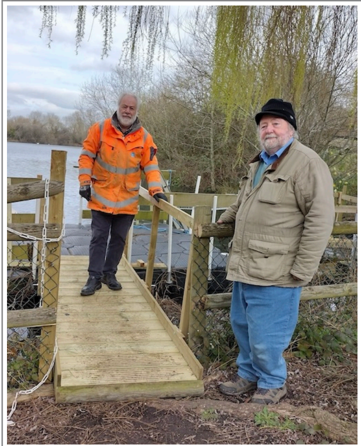
The new access ramp to the floating pontoon presented by Tony & Lawrie prior to the handover ceremony
